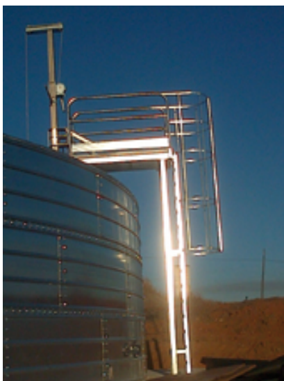
OVERHEAD SUPPORT FOR ELEVATED TANK That does not allow support on walls
